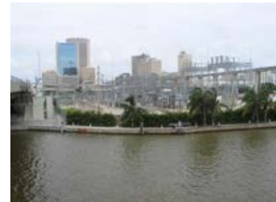
Existing: FPL Substation
